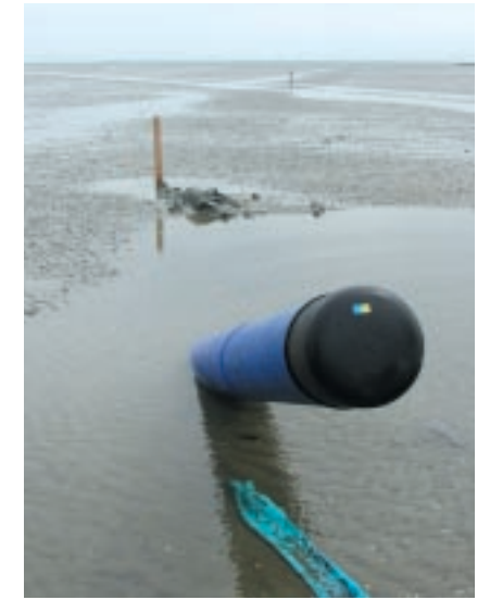
The pipe end in the mud-flats, which were installed with the "plow"
