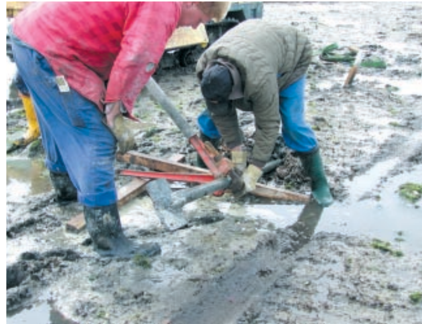
The bore head is exchanged for the backreamer with the attached PE pipe string.
