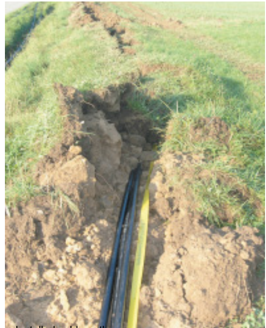
Installed cable path.
